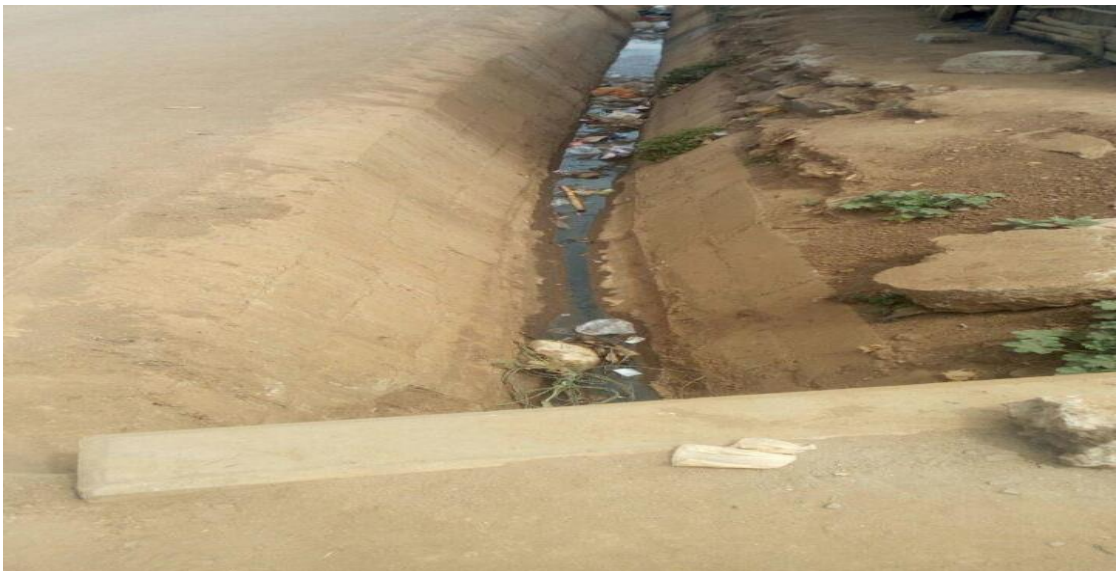
Figure 4.25 Storm Water Drainage in Kamukunji
