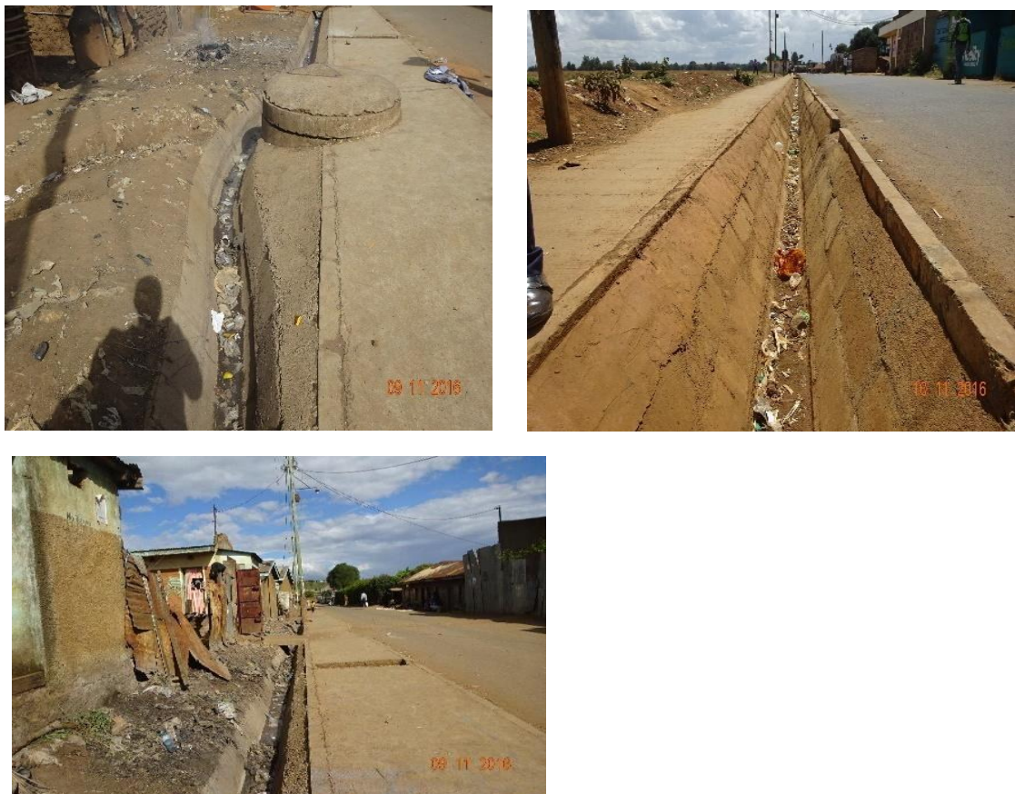
Figure 4.34: Some Unmaintained Drainage Systems in the Settlements
