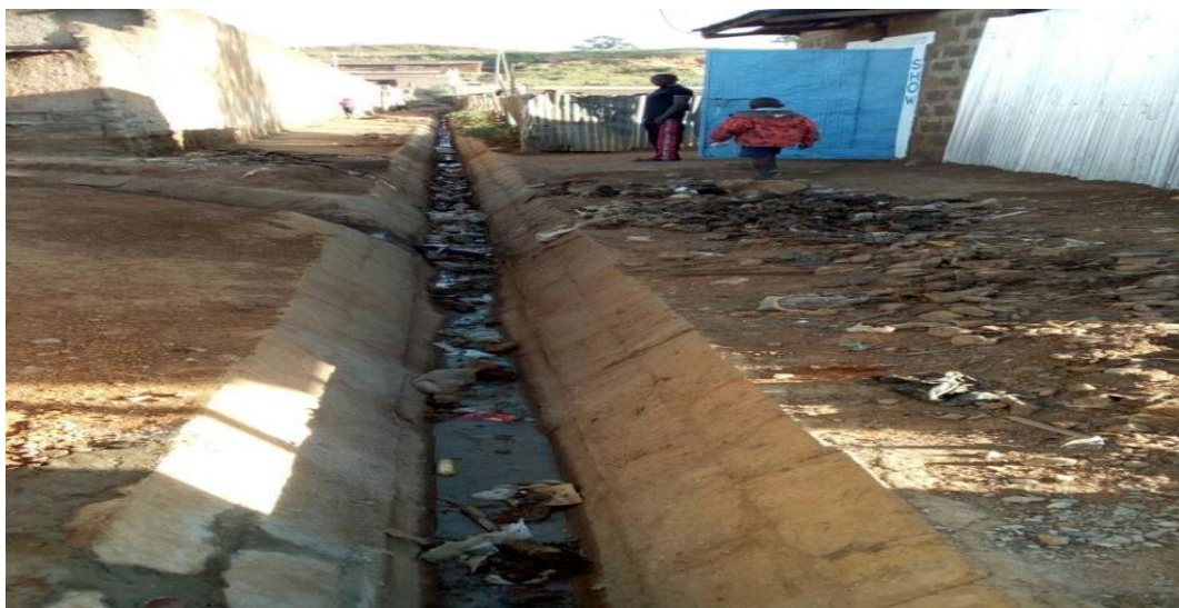
Figure 4.26: Poorly maintained drainage in Munyaka
