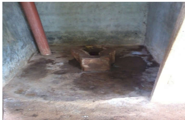
Figure 1: A Sullied Adapted Toilet with no Holding Rails
